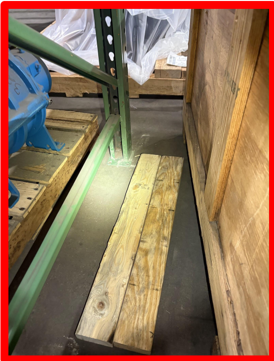
1CE, Bay 5 Upright Missing Anchors 4
