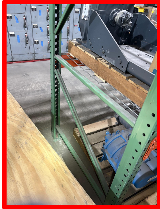
1CE, Bay 5 Upright Missing Anchors 4
