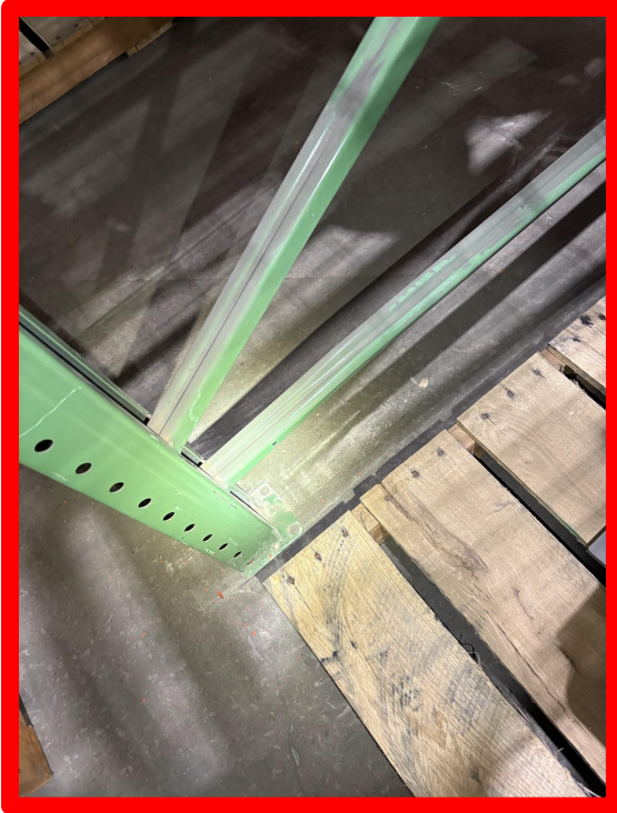
1CE, Bay 4 Upright Missing Anchors 4
