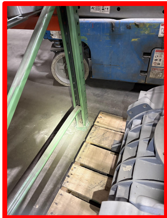
1CE, Bay 3 Upright Missing Anchors 4
