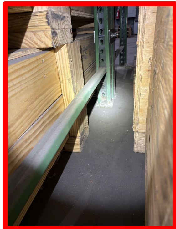
Row 1CB, Bay 5 Upright Missing Anchors 4
