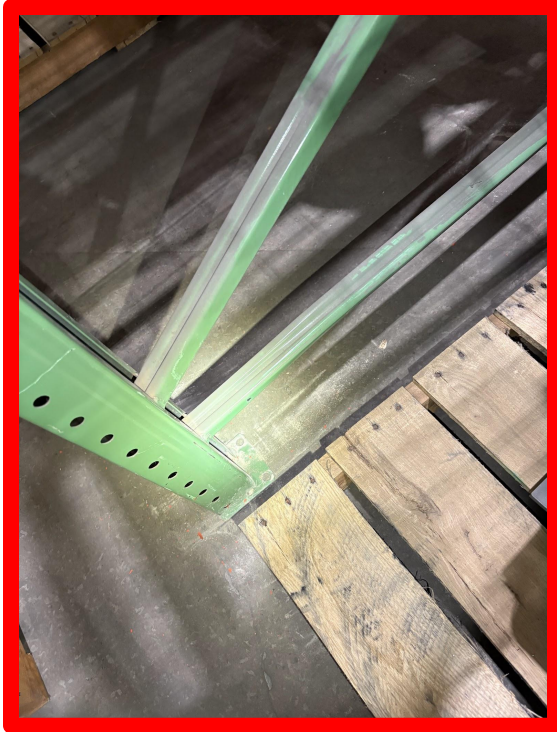
1CE, Bay 4 Upright Missing Anchors 4
