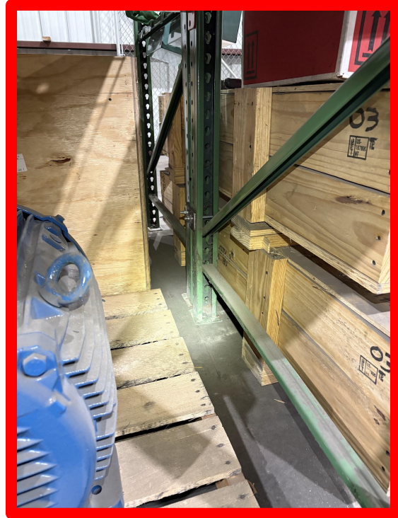
1CC, Bay 5 Upright Missing Anchors 4
