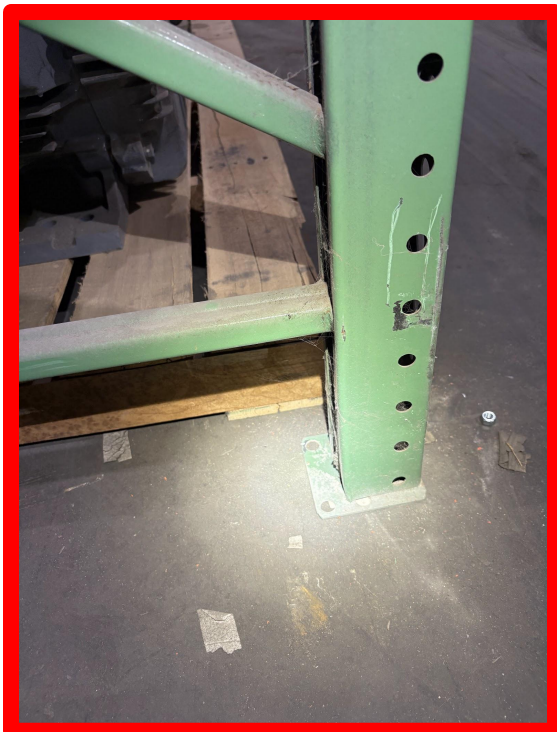
1CC, Bay 4 Upright Missing Anchors 4
