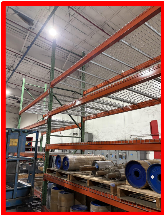
1CE, Bay 3 Beam Damage 3
