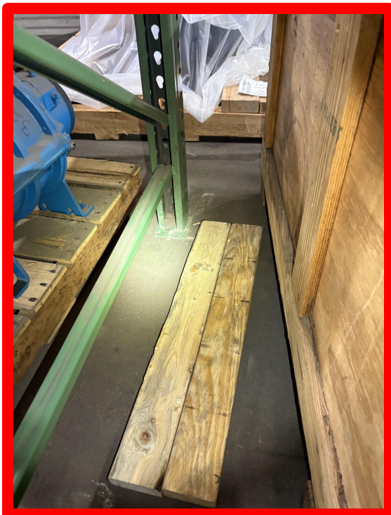
1CE, Bay 5 Upright Missing Anchors 4
